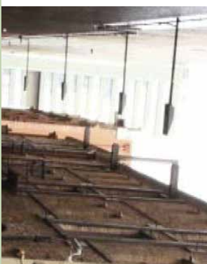
Fig. 7.3134 Wall Mounted Lighting
